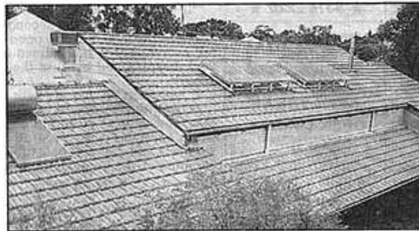
◆ The panels keep a low profile on the roofline.
